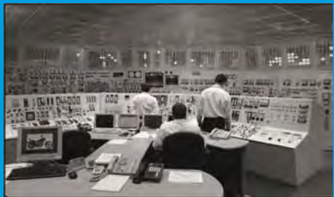
Conventional nuclear power plant control room
